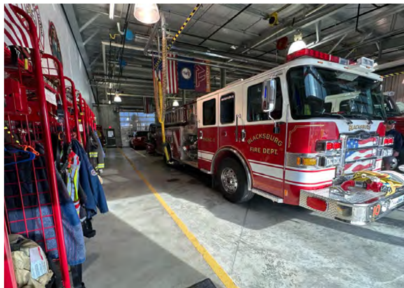
Diesel exhaust system in Blacksburg Fire Station
