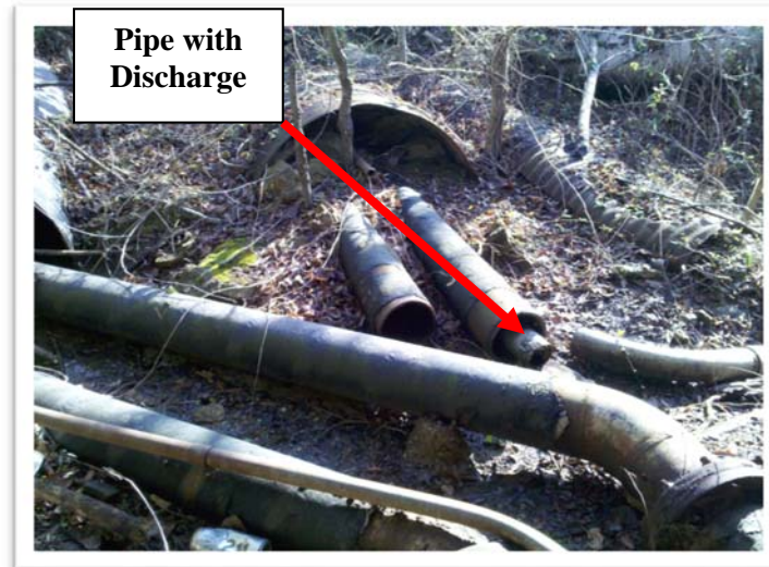
“Big Picture” photo shows pipe and surrounding layout.
