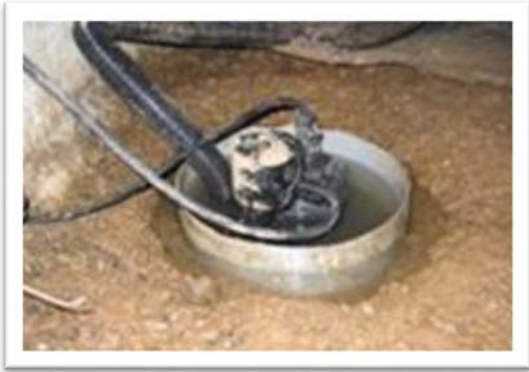
Basement/Crawlspace Sump Pumps
