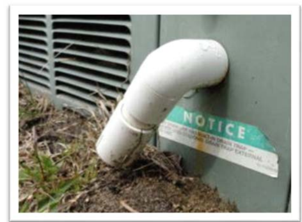
Air Conditioning Condensation
